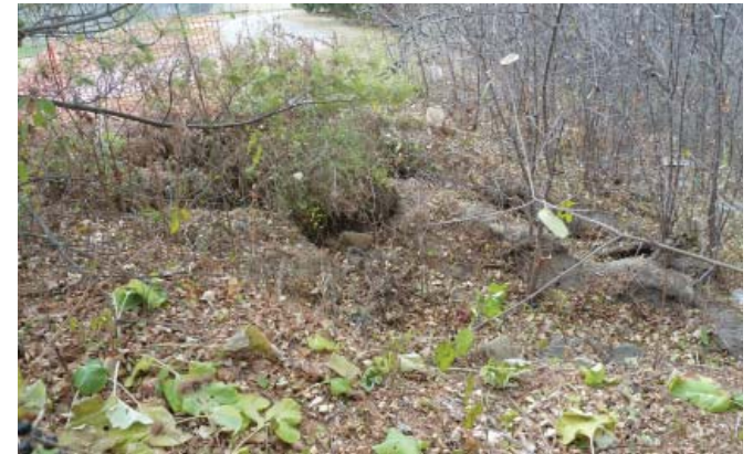
Erosion along the drainage way.
