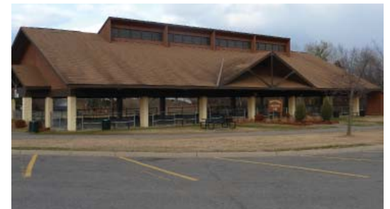
Roof drainage is causing flooding on the south side of the pavilion.
